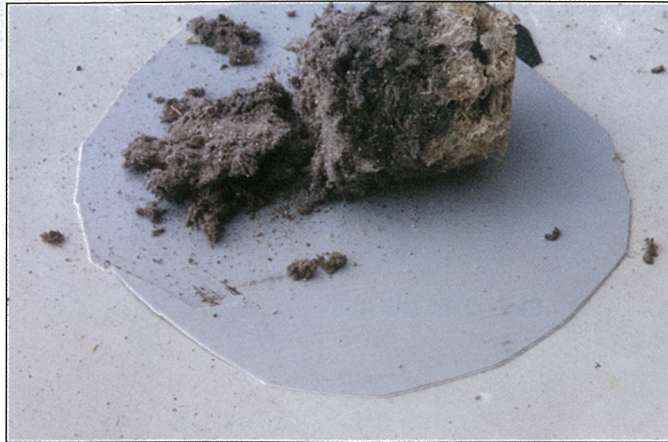
Core cuts show dry insulation.
